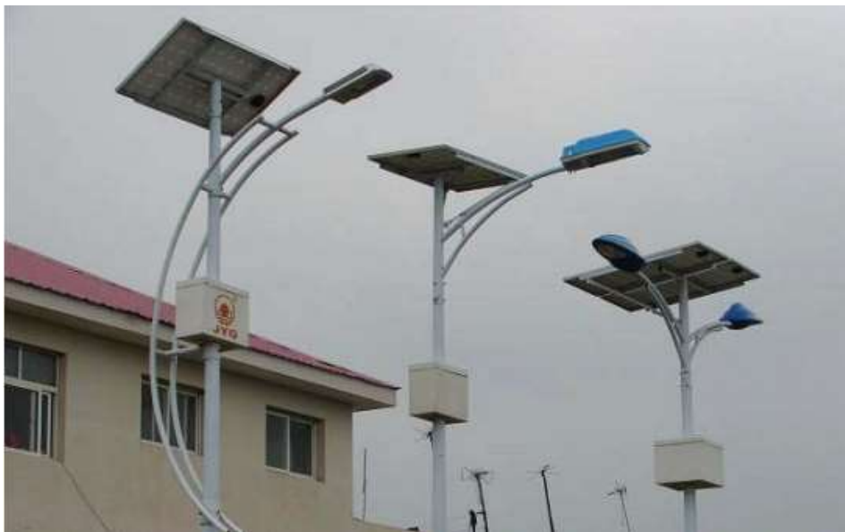
Gambar 4. Lampu PJU tenaga surya
